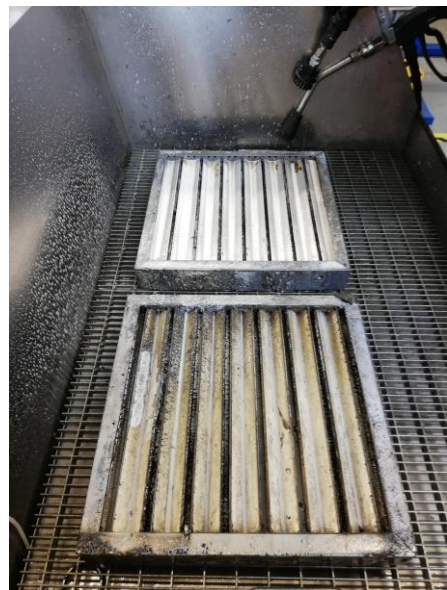
Grease filter in collector of 1000 SR front full of oil and grease, back cleaned
