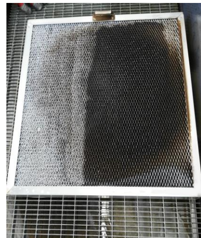
Oil filter: Left crudely cleaned, right uncleaned
