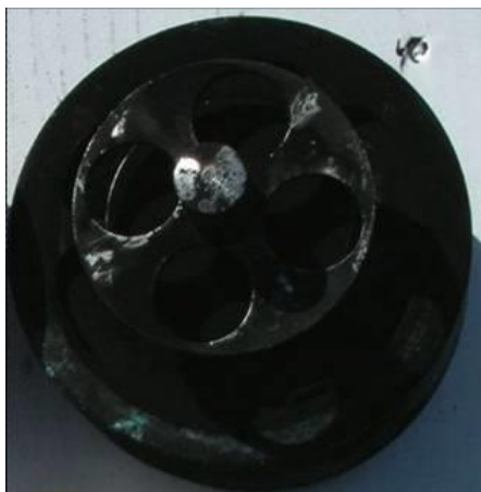
Soot filter uncleaned
